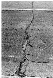
Gambar 2. 5 Retak Sambung ( Joint Reflection Cracking )
