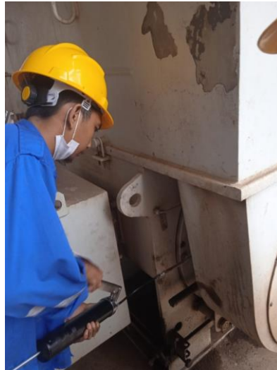
Gambar 2.32. PM Diarea Boiler
