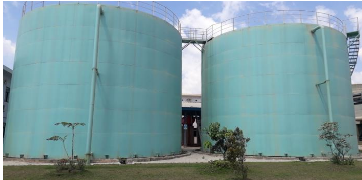
Gambar 2.18. Demin Tank PLTU Tenayan
