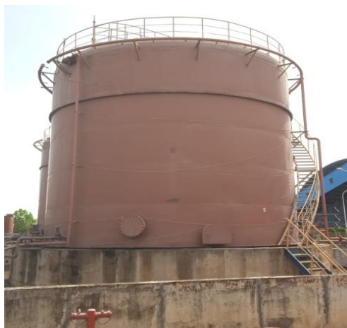
Gambar 1.28. Fuel Oil Tank PLTU TENAYAN
