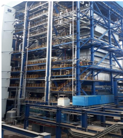
Gambar 2.2 Boiler PLTU Tenayan
