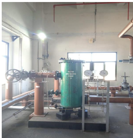
Gambar 2.30. Filter Unloading Pump 2 PLTU TENAYAN
