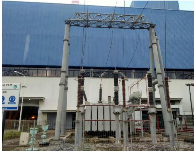
Gambar 2.10. Service Station Transformator (Sumber: Dokumentasi di PLTU TENAYAN)
