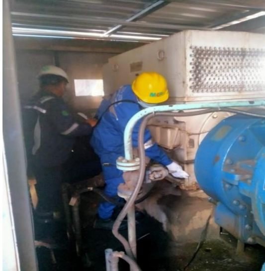
Gambar 1.36. PM Diarea Boiler Motor HPFF Unit 1
