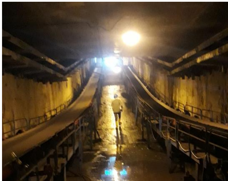
Gambar 2.22. Belt Conveyor PLTU Tenayan
