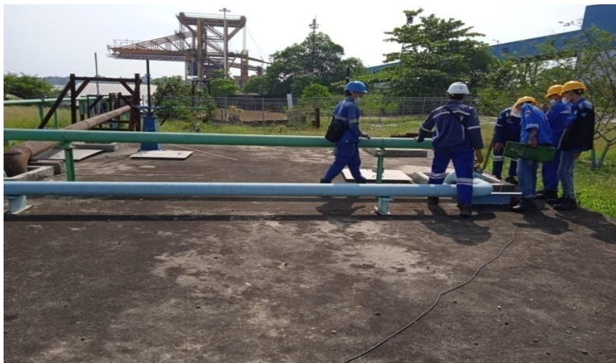
Gambar 2.14. Water Basin PLTU Tenayan (Sumber: Dokumentasi di PLTU TENAYAN)
