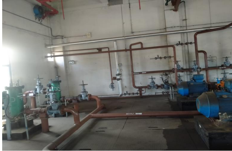
Gambar 2.31. Filter Supply Pump 1 dan 2 PLTU TENAYAN
