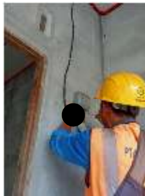
Gambar 2.11 pergantian MCB (main circuit braker)
