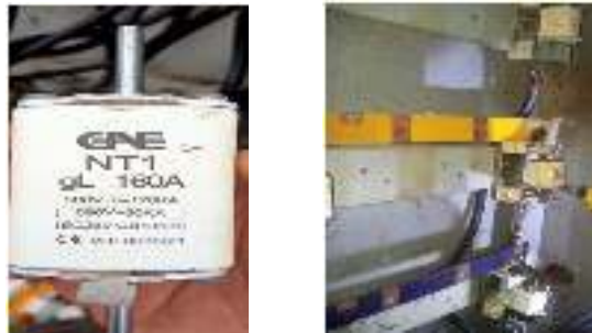
Gambar 2.21 pergantian NH Fuse ( Sumber : PT. Adra gemilang, 2023)
