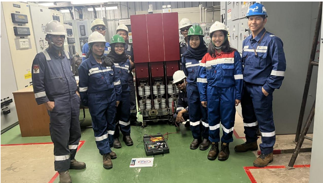
Gambar 2. 1 Preventive Meaintenance Breaker
