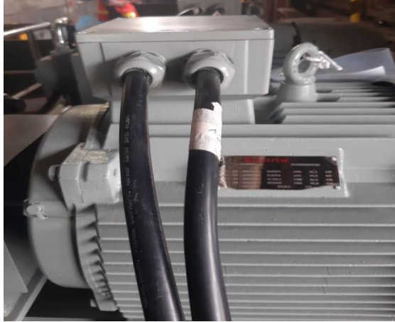
Gambar 2.7 Konek Kabel Power Motoran 3 Phasa Sumber : PT. Wilmar Nabati Indonesia Dumai-Pelintung, (2022)
