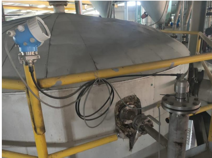
Gambar 3.3 Level transmitter di tangki Crystallizer Sumber : PT. Wilmar Nabati Indonesia Dumai-Pelitung, (2022)
