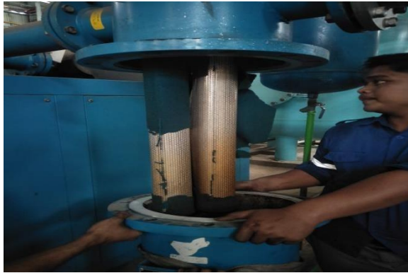
Gambar 2. 42 Pengecekan Filter Dryer (Sumber: Dokumentasi di PT. Indah Kiat Pulp and Paper)
