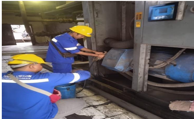
Gambar 2. 26 Greasing Motor Compressor (Sumber: Dokumentasi di PT. Indah Kiat Pulp and Paper)
