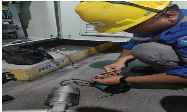
Gambar 2. 28 Test Motor Vale Compressor PG 2 (Sumber: Dokumentasi di PT. Indah Kiat Pulp and Paper)
