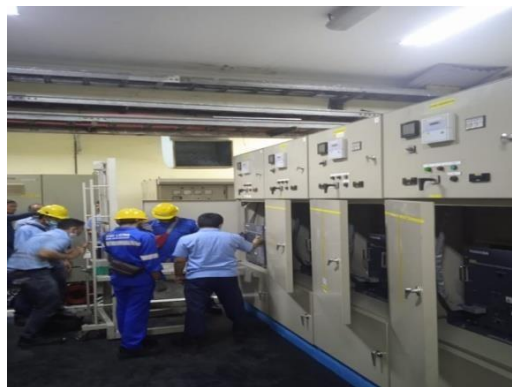
Gambar 2. 14 Cleaning Panel Compressor WT 1 (Sumber: Dokumentasi di PT. Indah Kiat Pulp and Paper)
