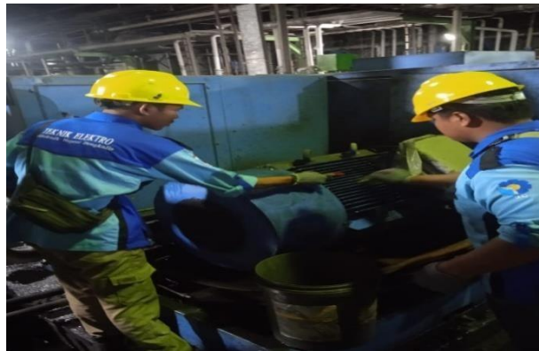
Gambar 2. 15 Cleaning Body Motor Compressor PG 2 (Sumber: Dokumentasi di PT. Indah Kiat Pulp and Paper)
