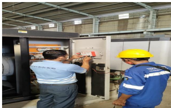
Gambar 2. 27 Greasing Motor Compressor (Sumber: Dokumentasi di PT. Indah Kiat Pulp and Paper)
