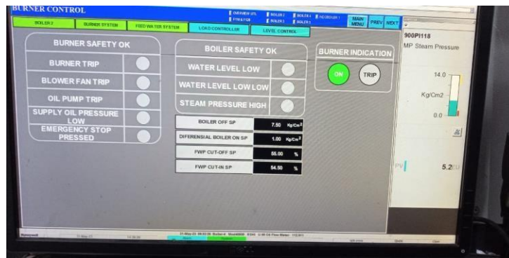
Gambar 3.4 System Burner Control
