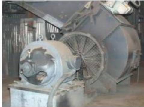
Gambar 3.17 Force Draft Fan Boiler
