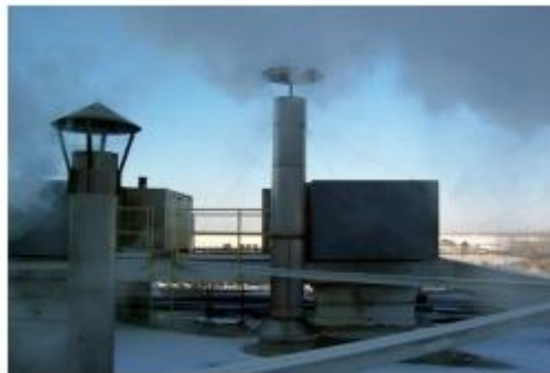
Gambar 3.20 Stack (Cerobong) Boiler
