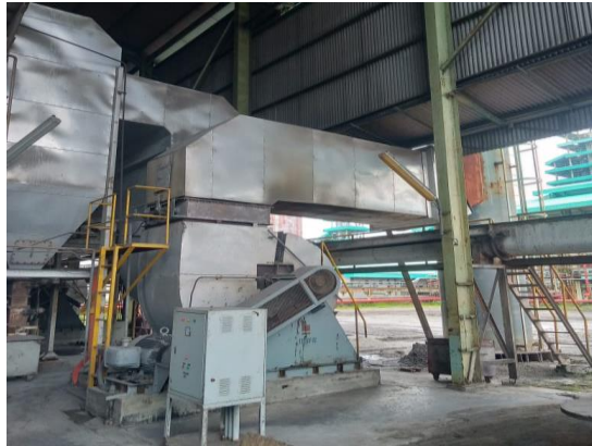
Gambar 4. 7 Induced Draft (ID) Fan (Sumber :dokumentasi penulis)
