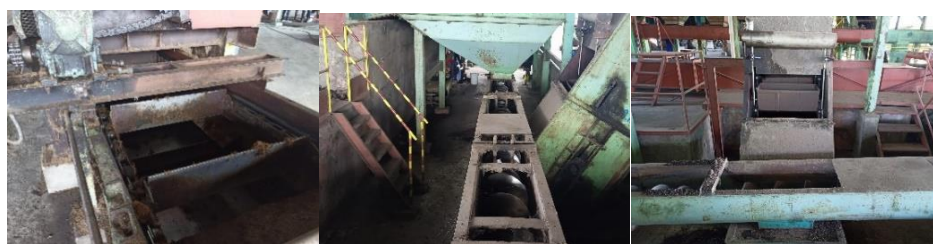
Gambar 4. 1 scraper conveyor, screw conveyor dan bucket elevator conveyor.
