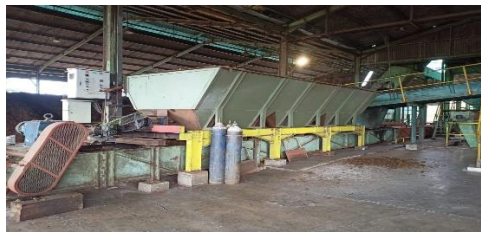
Gambar 4. 2 Area scaper conveyor 135. 3G. 09
