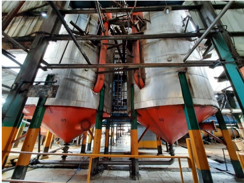
Gambar 2.13 Vertical Clarifier Tank (VCT) Sumber: PTPN V KEBUN TANAH PUTIH
