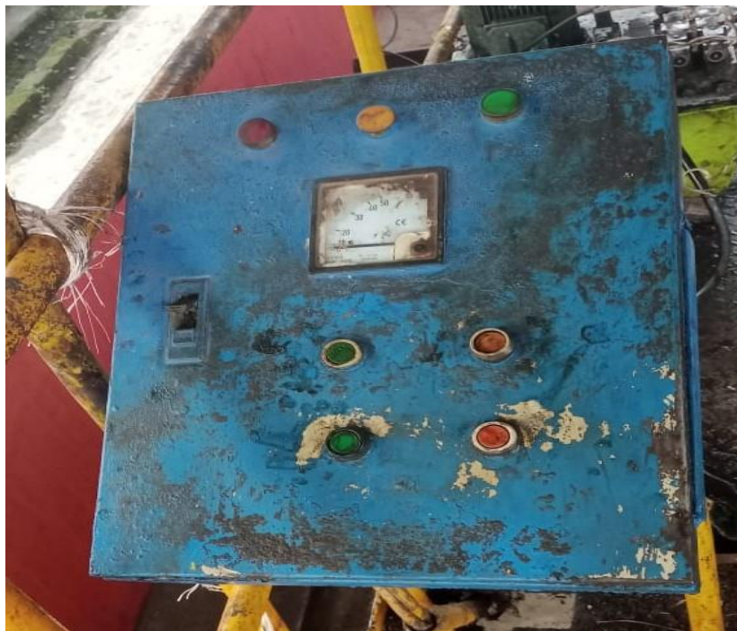
Gambar 3.23 panel pengendali Transfer Carriage
