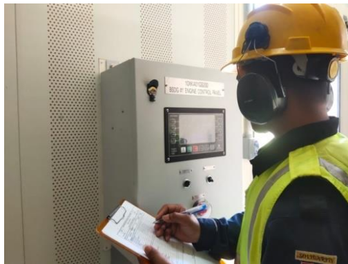
Gambar 3. 3 Weekly inspection Black Start Diesel Generator (BSDG 1)
