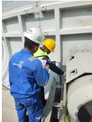
Gambar 3.4 Weekly Inspection Cooling Tower (Sumber : Dokumentasi pribadi)
