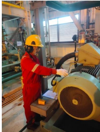
Gambar 3. 2 Weekly Inspection Steam Turbine Generator (STG)
