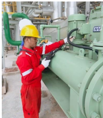
Gambar 3.5 Weekly Inspection Head Recovery Steam Generator (STG) (Sumber : Dokumentasi pribadi)
