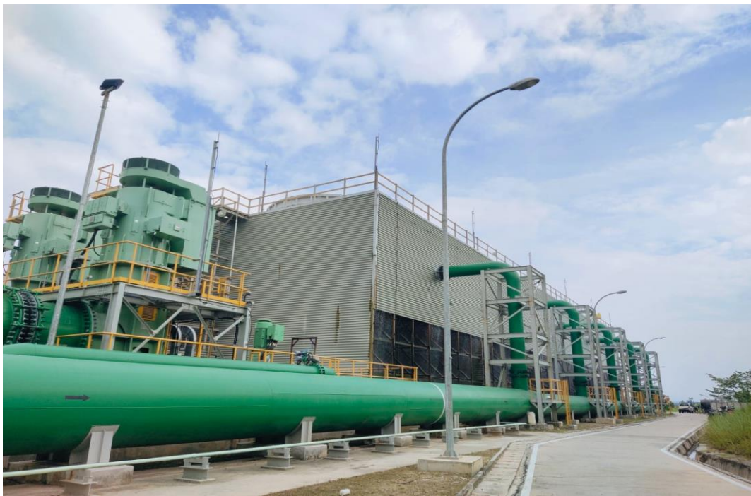
Gambar 4. 1 Cooling Tower (Sumber :dokumentasi pribadi)
