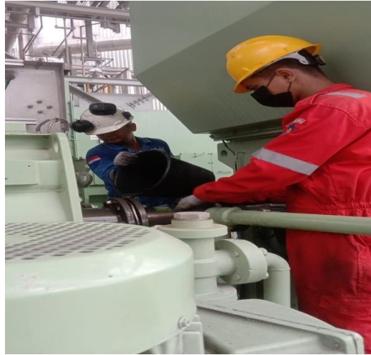
Gambar 3. 4 PM Boiler Feed Water Pump
