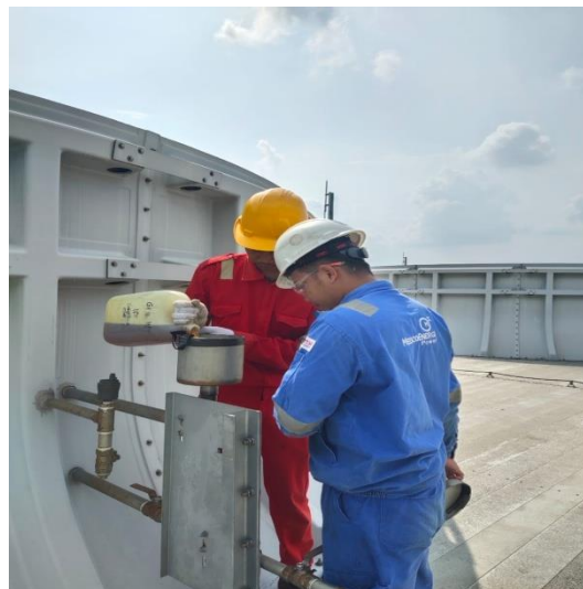
Gambar 3. 5 PM Cooling Tower
