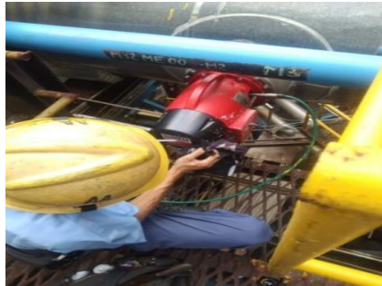
Gambar 2. 6 Cleaning Sensor Consistency Di PD10 (Sumber: Dokumentasi PT. Indah Kiat pulp & paper Tbk Perawang, 2023)
