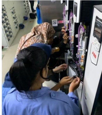
Gambar 2. 14 Memastikan Variable Speed Driver keadaan off
