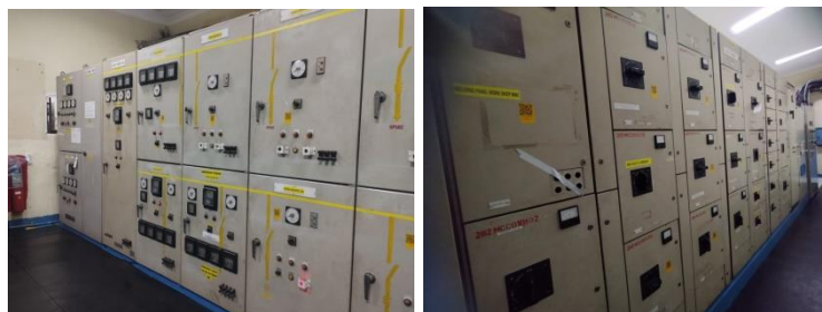
Gambar 3. 5 Main Control Center
