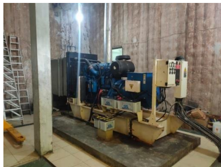
Gambar 4.2 Mesin Emergency Diesel Generator (Sumber: dokumen pribadi)
