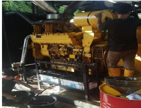
Gambar 2.12 Servis mesin unit 5 (Sumber : PT.Megapower Makmur Tbk,2023)
