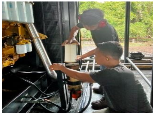
Gambar 2.11 Servis mesin unit 5 (Sumber : PT.Megapower Makmur Tbk,2023)
