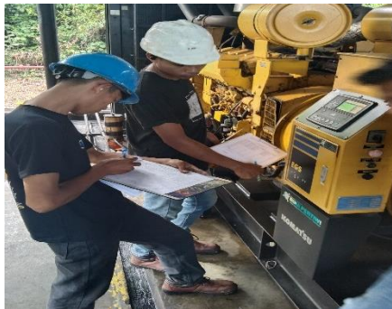
Gambar 2.20 Monitoring kWh (Sumber : PT.Megapower Makmur Tbk,2023)
