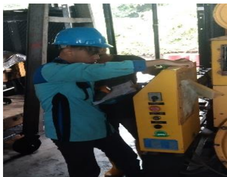
Gambar 2.16 Monitoring kWh (Sumber : PT.Megapower Makmur Tbk,2023)
