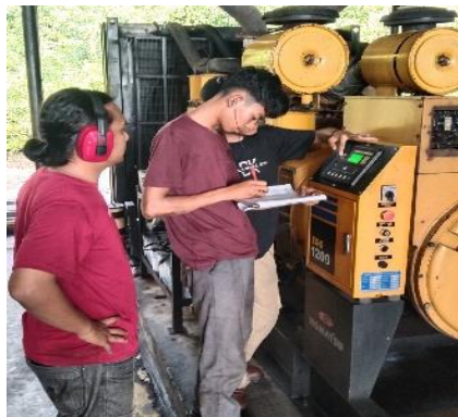
Gambar 2.4 Monitoring kWh (Sumber : PT.Megapower Makmur Tbk,2023)
