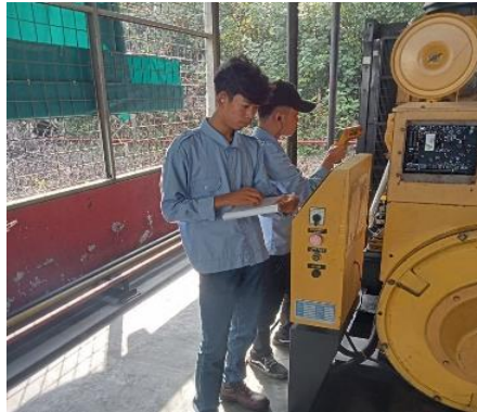
Gambar 2.3 Monitoring kWh (Sumber : PT.Megapower Makmur Tbk,2023)
