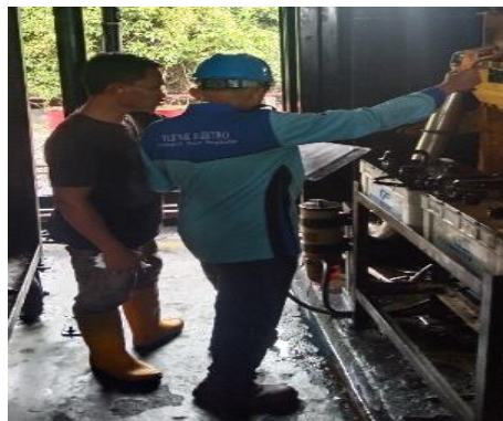
Gambar 2.5 Monitoring kWh (Sumber : PT.Megapower Makmur Tbk,2023)
