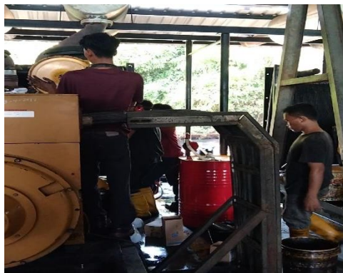
Gambar 2.17 Mengganti filter (Sumber : PT.Megapower Makmur Tbk,2023)
