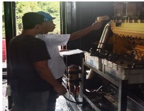
Gambar 2.13 Monitoring kWH (Sumber : PT.Megapower Makmur Tbk,2023)
