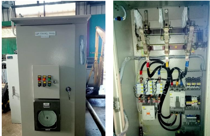
Gambar 4.3 panel control esp
