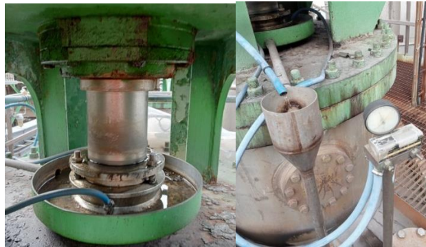
Gambar 4.21. Kondisi Sealing Water Critical Gearbox
