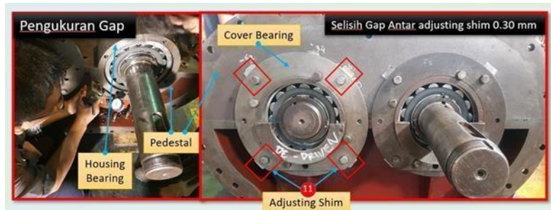
Gambar 4. 7 mengukur gap pedestal to cover housing bearing, Sumber. INSTRUKSI KERJA (IK) PJB-IMS 2.0
