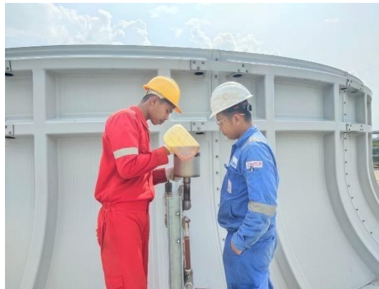
Gambar 3.5 PM Cooling Tower (Sumber : Dokumentasi Pribadi)
