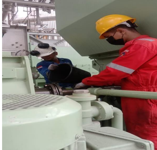
Gambar 3.4 PM Boiler Feed Water Pump (Sumber : Dokumentasi Pribadi)
