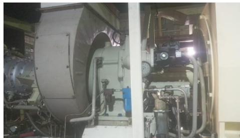
Gambar 4.3: Gearbox Turbin Generator
