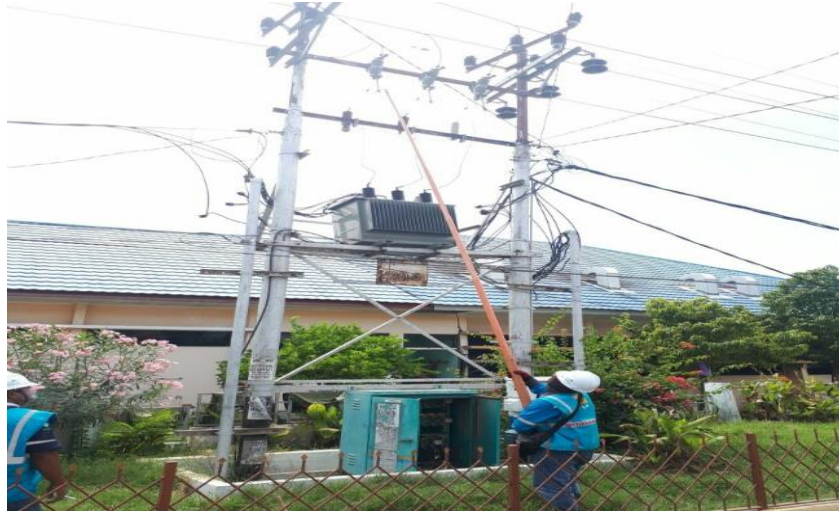
Gambar 3. 1 gardu distribusi pln dumai
