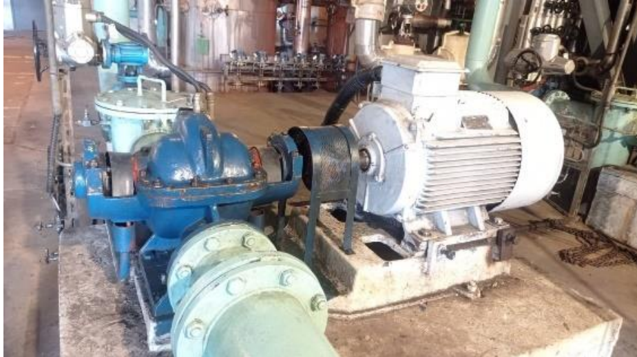
Gambar 4.1 Pompa Close Cycle Cooling Water (Sumber : Dokumentasi Pribadi)
