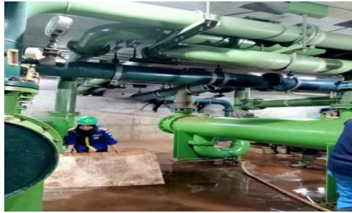
Gambar 2.2 Heat Exchanger 1 dan unit 2
