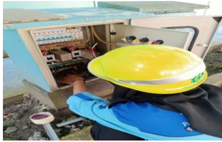
Gambar 2.26 Tranducer dan panel Pompa IPAL
