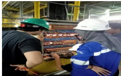
Gambar 2.51 Panel oil pumping set control unit 2
