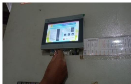
Gambar 2.37 Monitor HMI RTD
