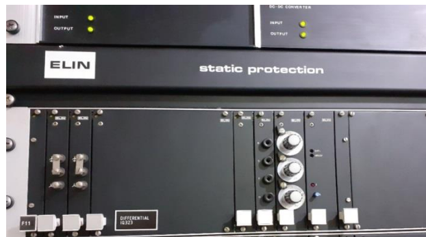
Gambar 4.3 Panel Relay Differential unit 2 ULPLTA Koto Panjang
