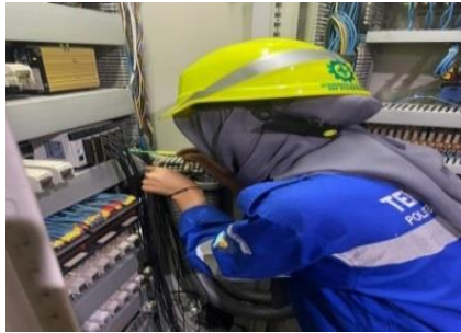
Gambar 2.32 RTD panel generator control unit 3
