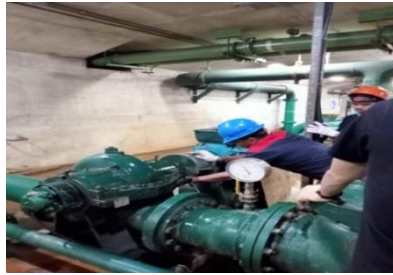
Gambar 2.56 Pompa raw water
