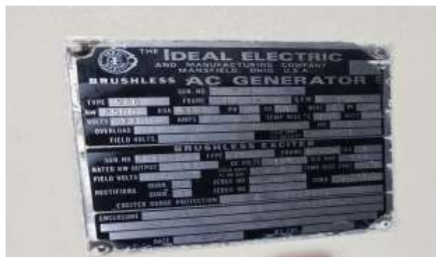
Gambar 3.4 Name Plate Generator
