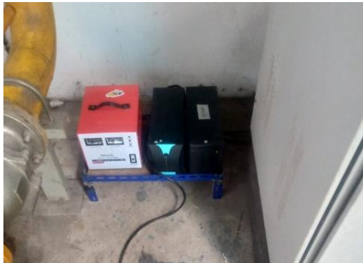
Gambar 2.72 UPS ( Uninterruptible Power Supply ) Sumber: (Dokumentasi, 2023)
