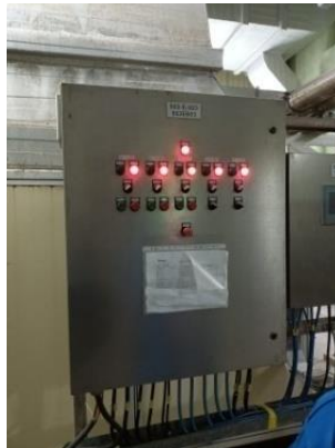
Gambar 2.44 Pengecekan AHU Panel
