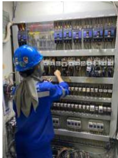
Gambar 2.32 Pengecekan Panel MCC
