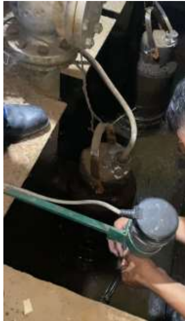
Gambar 2.4 Maintanance Level Switch
