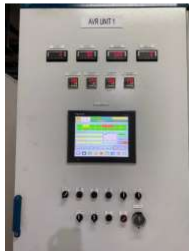
Gambar 4.10 Panel AVR Unit 1
