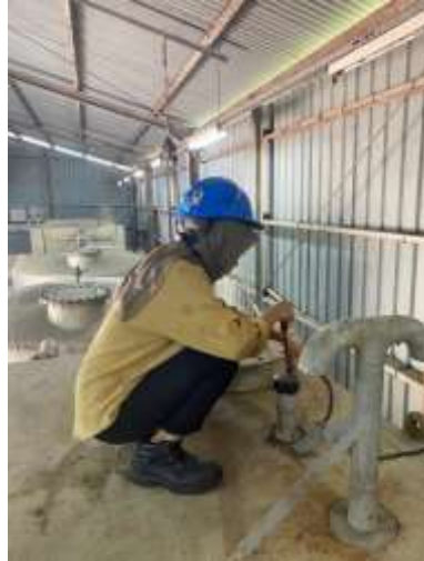
Gambar 2.21 Maintanance level switch
