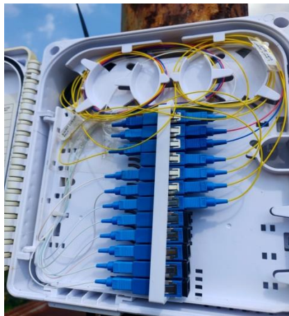
Gambar 4.3 Optical Distribution Point (ODP)
