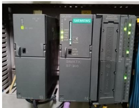
Gambar 3.9 PLC Simens S7-300
