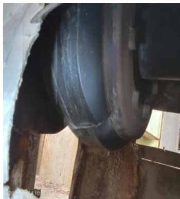
Gambar 4.19 Coupling rusak Sumber : Fiberline 2#, PT. RAPP
