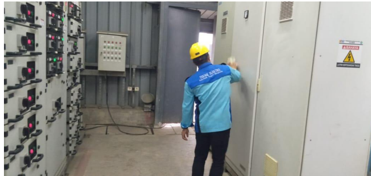
Gambar 2.36 Preventive Maintenance (PM) (Sumber: Dokumentasi 2023)
