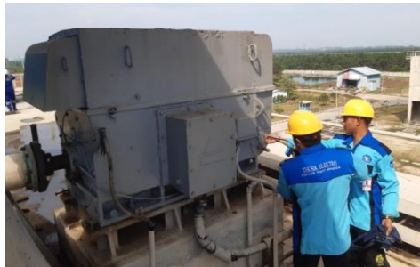
Gambar 2.6 Regreasing colling tower (Sumber : Dokumentasi 2023)
