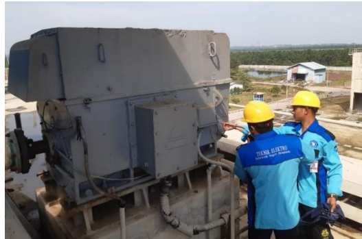
Gambar 2.8 Regreasing colling tower (Sumber : Dokumentasi 2023)
