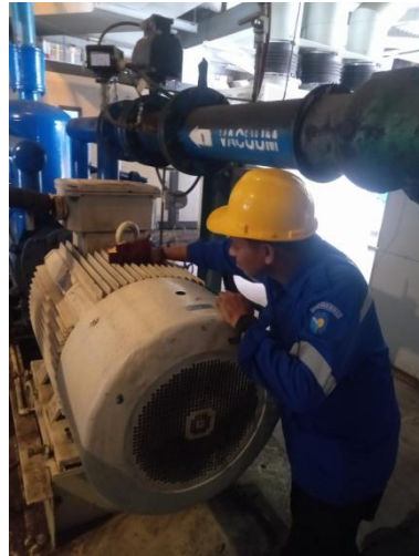
Gambar 2.44 Preventive Maintenance PLTU ROTARY COOLER BOTTOM ASH
