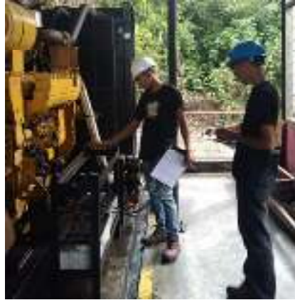
Gambar 2.44 Kegiatan monitoring KWH (Sumber: PT. Megapower Makmur Tbk, 2023)
