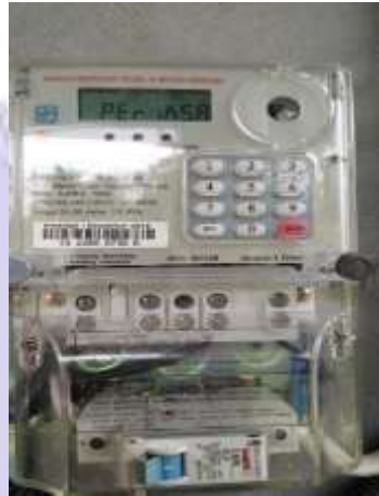
Gambar 2.8 kwh meter periksa
