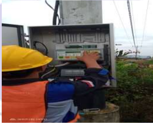
Gambar 3.1 .panel box recloser
