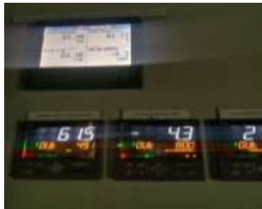
Gambar 2. 23 Monitoring Level Air di drum boiler Sumber : Dokumentasi 2023
