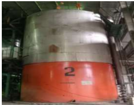
Gambar 3. 7 Continius Oil Tank Sumber : Dokumentasi 2023
