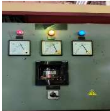
Gambar 4. 7 Panel Bank Capacitor
