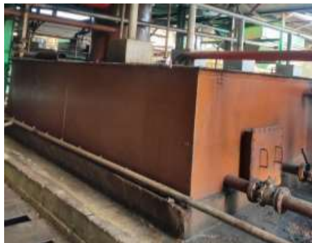
Gambar 3. 6 Crude Oil Tank Sumber : Dokumentasi 2023
