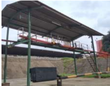
Gambar 3. 13 Oil Loading Sheet Sumber :Dokumentasi 2023
