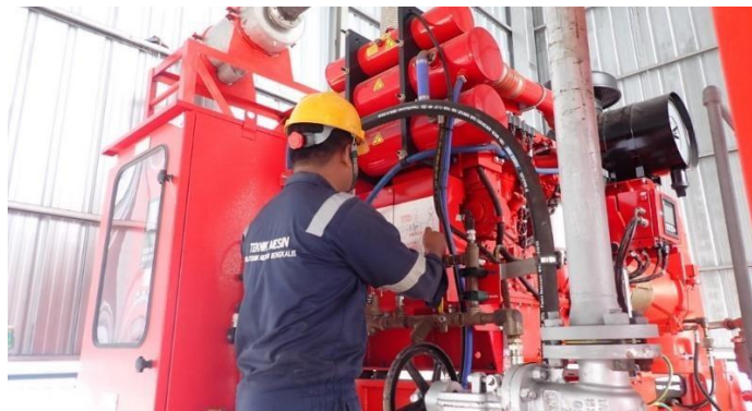
Gambar 3.1 PM di area engine fire pump house jetty 1 marine (Sumber : Dokumentasi Pribadi)
