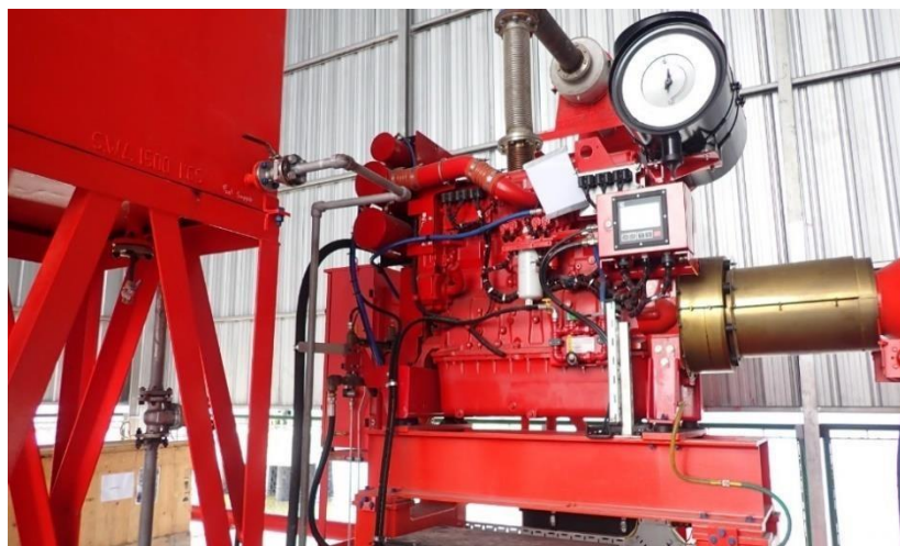
Gambar 4.2 FIRE PUMP 717-PE-3
