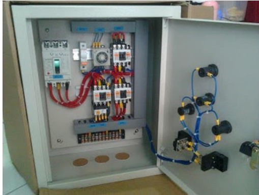
Gambar 3.16 Panel Listrik Sistem Interlock (Sumber: plcdroid ,2019)
