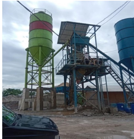
Gambar 4. 14 Batching plant pencampuran ready mix
