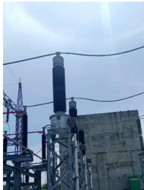
Gambar 3. 3 Capasitive Voltage Transformer (CVT) (Sumber : Dokumentasi,2023)
