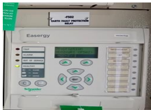
Gambar 3. 11 Ground Fault Relay (Sumber : Dokumentasi, 2023)
