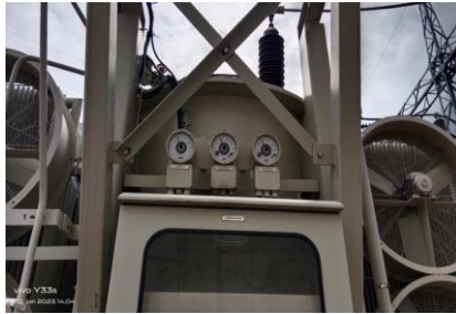
Gambar 3. 13 Relay HV/LV Winding Temperature (Sumber : Dokumentasi, 2023)
