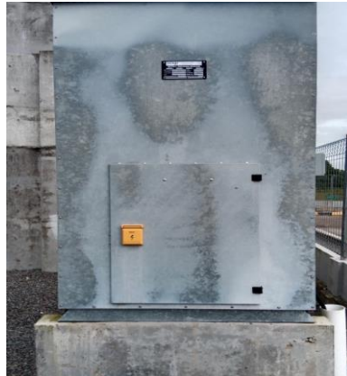
Gambar 3. 7 Neutral Grounding Resistance (NGR) (Sumber : Dokumentasi, 2023)
