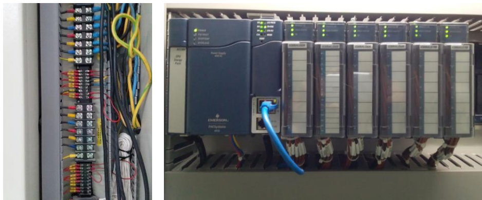
Gambar 2. 12 PLC Water Treatment Plant (Sumber : Dokumentasi, 2023)
