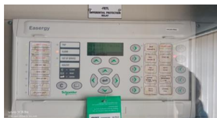
Gambar 3. 9 Differential Protection Relay (Sumber : Dokumentasi, 2023)
