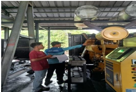
Gambar 2.20 Kegiatan monitoring KWH (Sumber: PT. Megapower Makmur Tbk, 2023)
