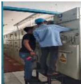
Gambar 2.20 Kegiatan monitoring KWH (Sumber: PT. Megapower Makmur Tbk, 2023)
