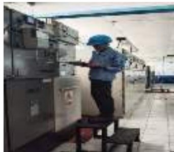
Gambar 2.2 Kegiatan monitoring KWh (sumber: PT. Megapower Makmur Tbk, 2023)
