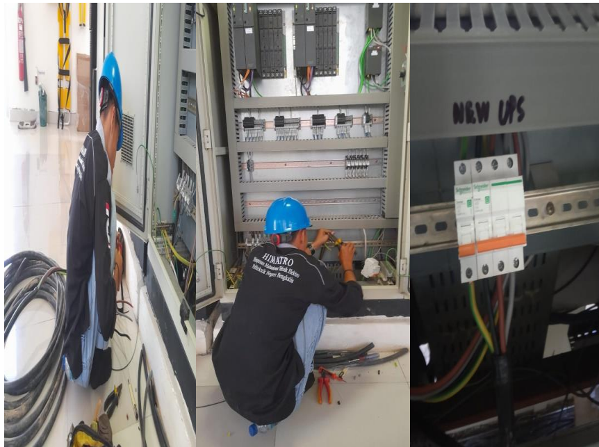
Gambar 2.3 pulling cabel and install power for UPS Sumber : Dokumen Perusahaan PT. Sari Dumai Oleo
