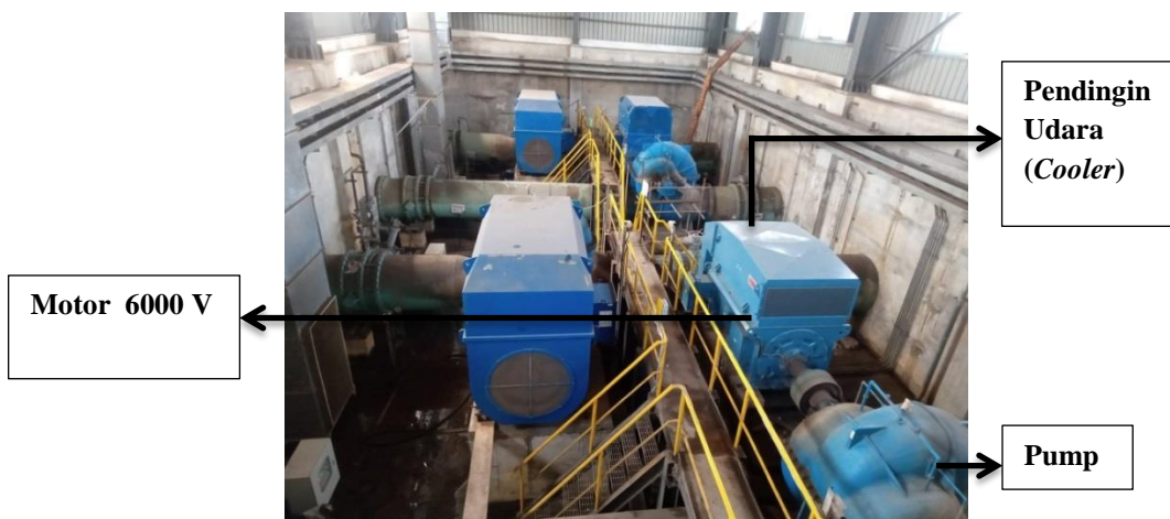
Gambar 3. 1 Motor Circulating Water Pump (CWP)
