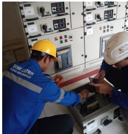
Gambar 2. 22 Proses pengecekan Braker Motor Intermediate (Sumber : Dokumentasi 2023)
