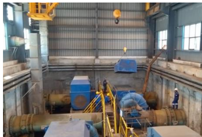
Gambar 2. 6 Proses Change over Cooler CWP (Sumber : Dokumentasi 2023)
