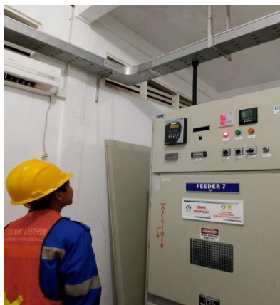
Gambar 2. 53 Pengecekan beban feeder Sumber: PT. Adra Gemilang. 2023
