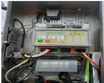
Gambar 2. 8 Pengecekan evidence dan recloser Sumber : PT. Adra Gemilang. 2023
