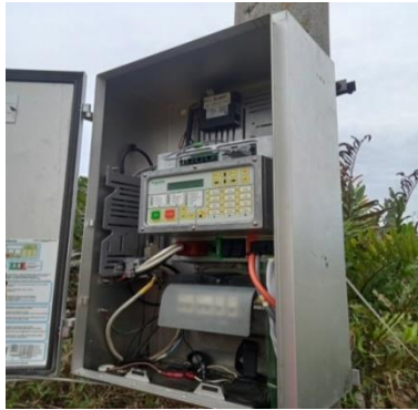
Gambar 2. 18 Penormalan recloser Sumber: PT. Adra Gemilang. 2023
