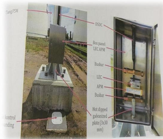
Gambar 2.28 Panel Monitoring LPS
