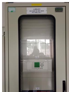
Gambar 2. 20 Remote Terminal Unit
