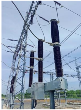
Gambar 2. 13 Circuit Breaker Line Trafo ( sumber :dokumentasi )
