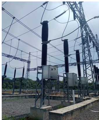
Gambar 3. 6 Circuit Breaker (CB) (Sumber :Dokumentasi,2023)
