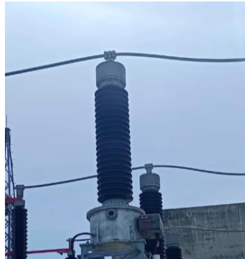
Gambar 3. 5Capacitive Voltage Transformer(CVT) (Sumber :Dokumentasi,2023)
