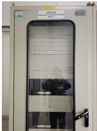
Gambar 2. 22 Panel 2 Substation Automation System (sumber :dokumentasi penulis)
