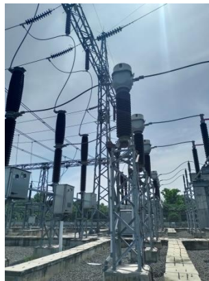
Gambar 3. 4 CT ( Current Transformer ) (Sumber : Dokumentasi,2023)
