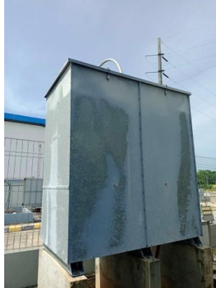
Gambar 3. 3 NGR ( Neutral Grounding Resistance ) (Sumber : Dokumentasi,2023)
