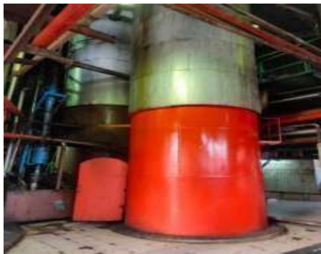
Gambar 2. 13 Oil Tank dan sludge tank
