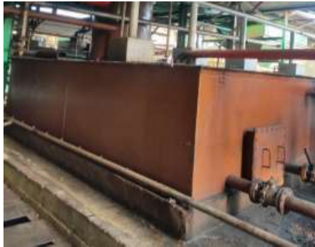
Gambar 2. 11 Cruide Oil Tank
