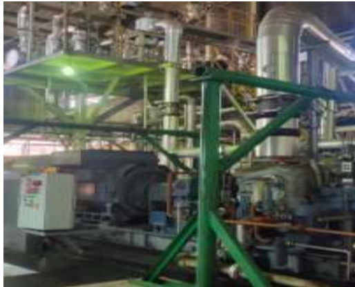
Gambar 2. 8 Power Plant Sumber Dokumentasi 2023
