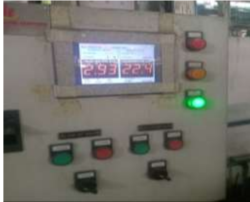
Gambar 2. 38 Monitoring Steam di power plant Sumber Dokumentasi 2023
