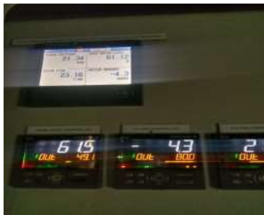
Gambar 2. 39 Monitoring Steam di Boiler Sumber Dokumentasi
