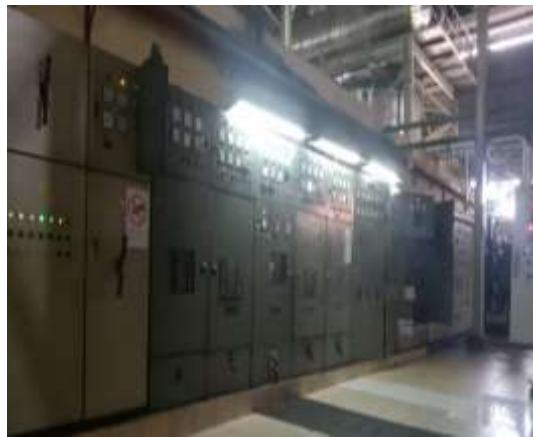
Gambar 2. 42 Monitoring di Power Plant Sumber Dokumentasi 2023
