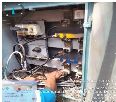
Gambar 2.41 Kegagalan isolasi kabel outgoing ke ground plate (Sumber PT.Haleyora Power 2023)
