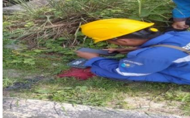
Gambar.2.47.pengukuran tegangan grounding travo (Sumber PT.Haleyora Power,2023)
