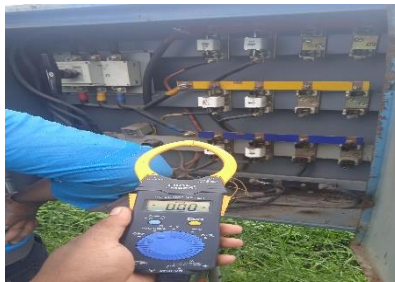
Gambar.2.24 Pengukuran trafo (Sumber PT.Haleyora Power,2023)
