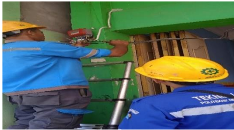
Gambar.2.4.Menganti KWh. (Sumber PT.Haleyora Power,2023.)
