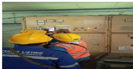
Gambar.2.27. Periksa GH (Sumber PT.Haleyora Power,2023)
